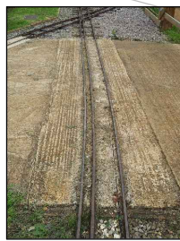
Detail B Typical arrangement of track bed at pedestrian and vehicular crossing points. Track to be cast in concrete with existing surface treatment graded into the edge of concrete to remove trip hazard.
